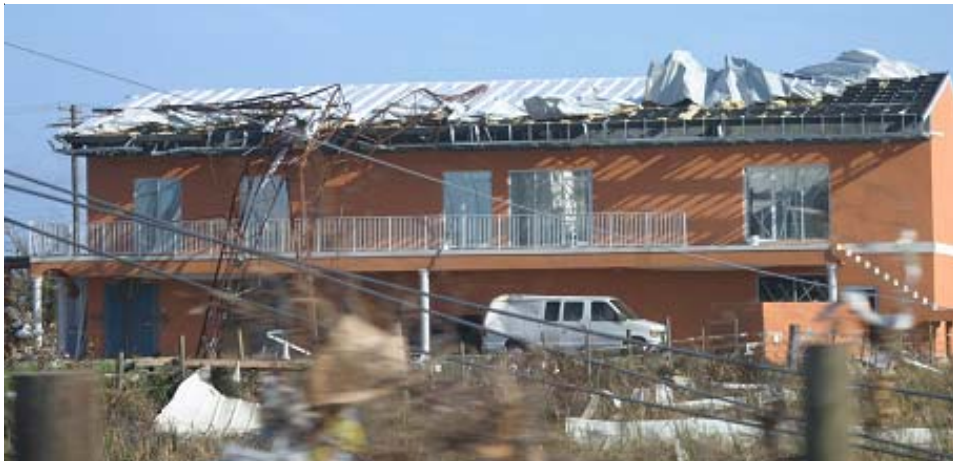
The importance of rebuilding to standard: This building's roof was ripped off by a piece of debris from another structure.
